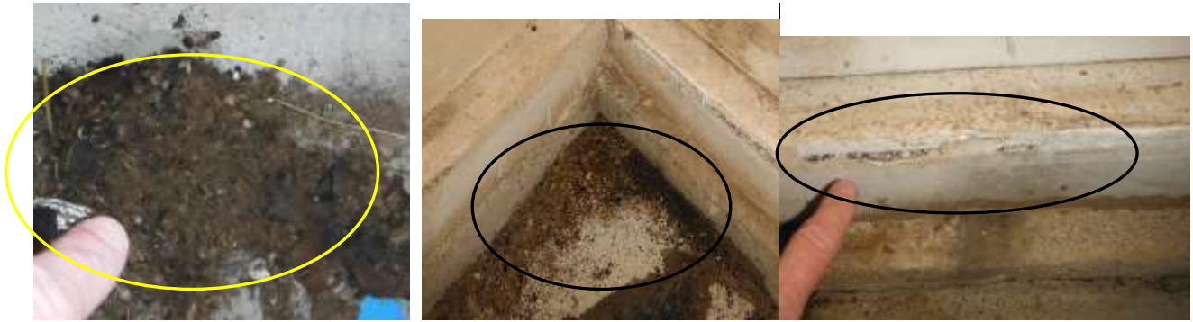
Figure 33 Carpenter ant frass/nest, damage, and chewed paper; have a licensed Pest Company treat for all wood destroying insects.
