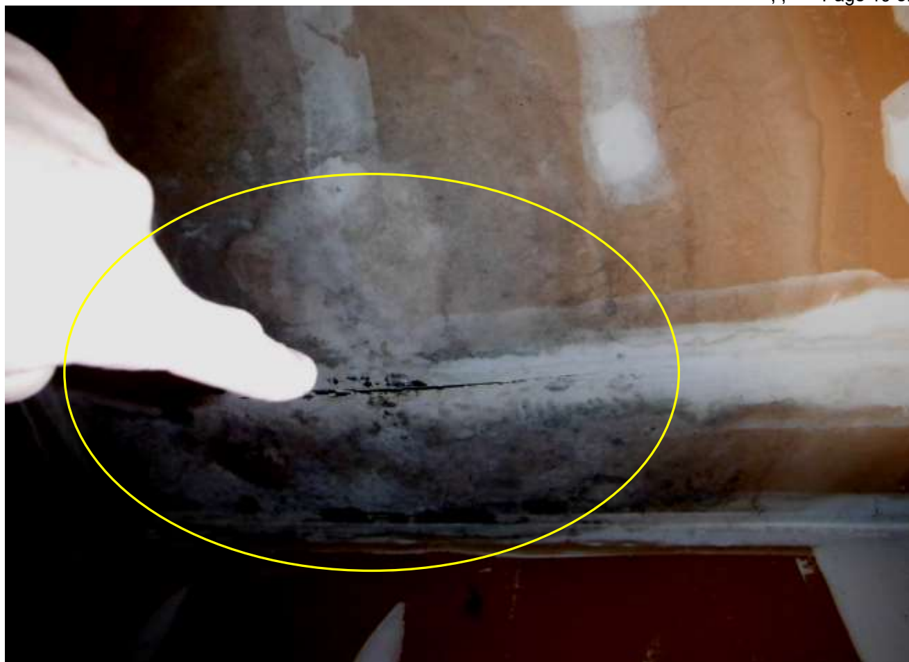
Figure 10 Example of roof leaking & water damage in garage. Have a structural carpenter evaluate extent of all damage including water, mold like staining & insect before closing. The home was poorly maintained and needs upgrades and repairs everywhere.
