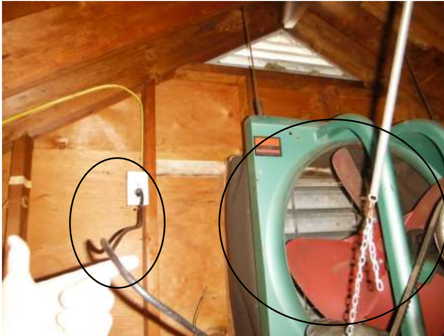
Figure 41 Attic fan had not grille and not wired with power switch; safety hazards.
