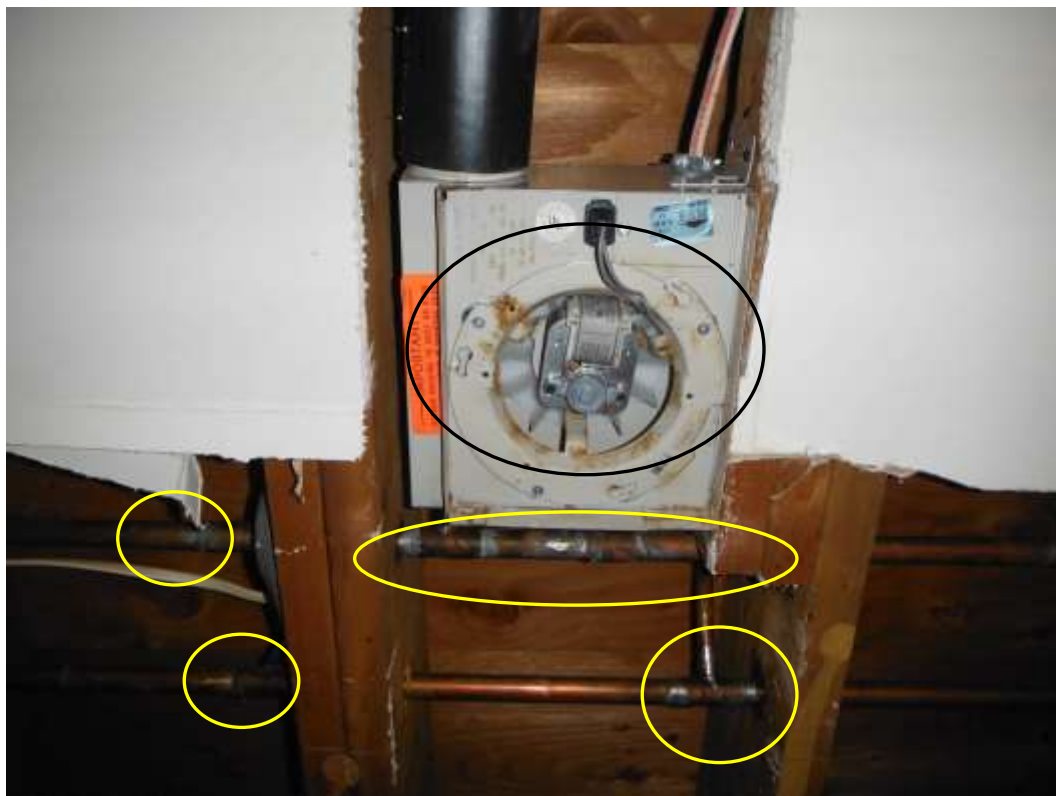
Figure 37 Opened ceiling and plumbing repairs; indication of frozen pipes/leak repairs. Have a bathroom contractor evaluate bathroom and upgrade with required permits.
