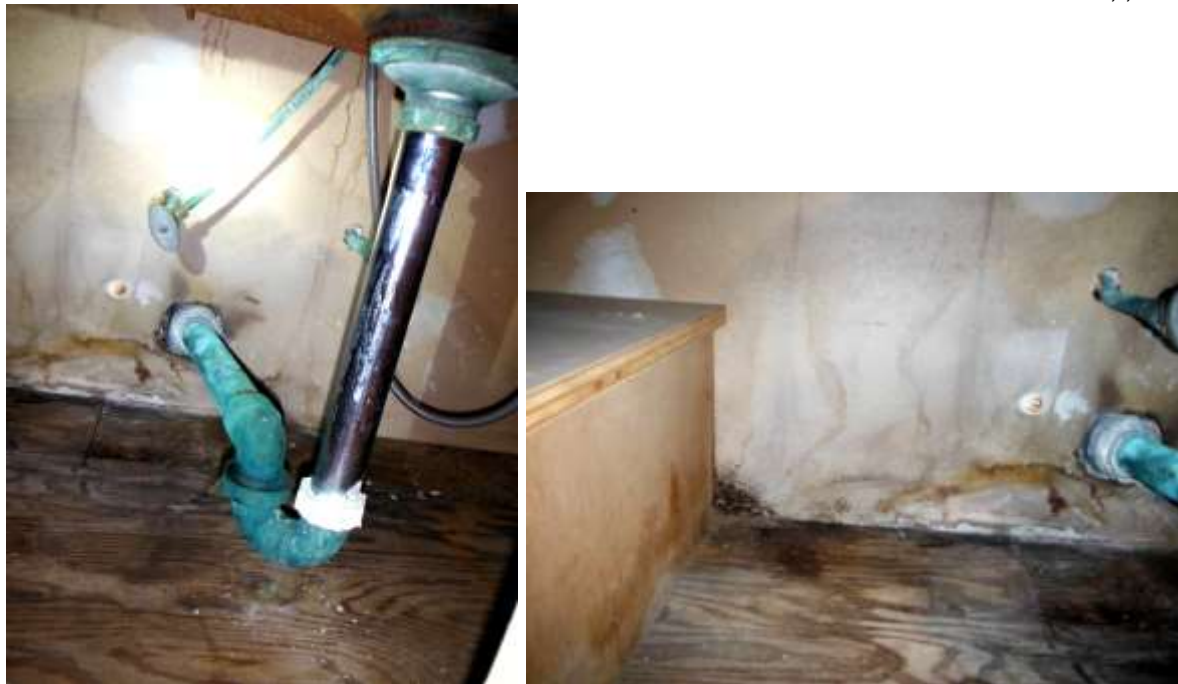
Figure 36 Leaking, corrosion, old plumbing; have licensed plumber evaluate for plumbing upgrades throughout the home.
