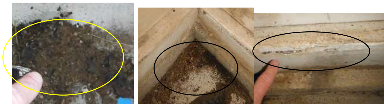
Figure 9 Carpenter ant frass/nest, damage, and chewed paper; have a licensed Pest Company treat for all wood destroying insects.
