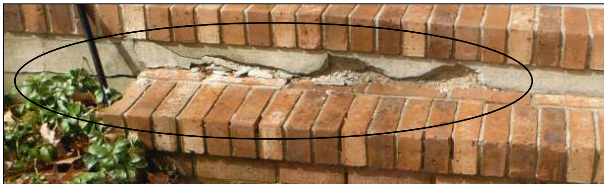
Figure 1 Have a mason evaluate/repair steps.
