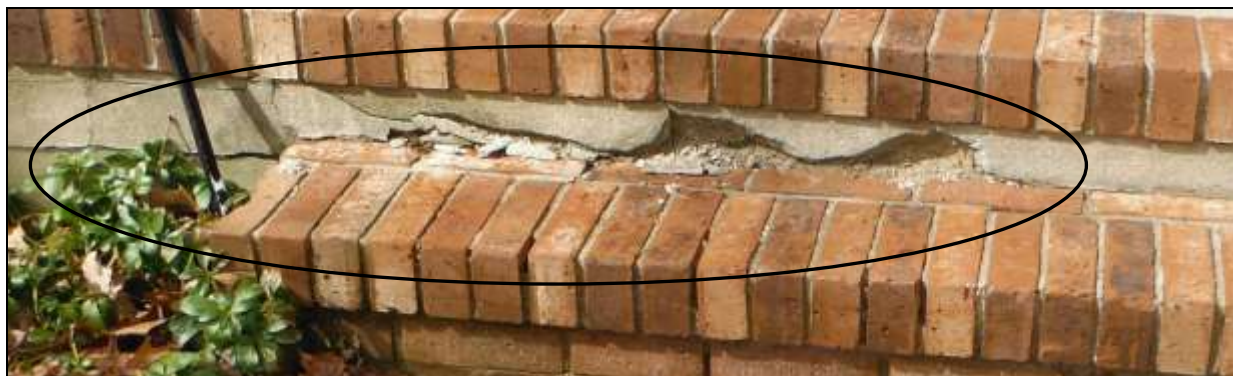
Figure 25 Have a mason evaluate/repair steps.
