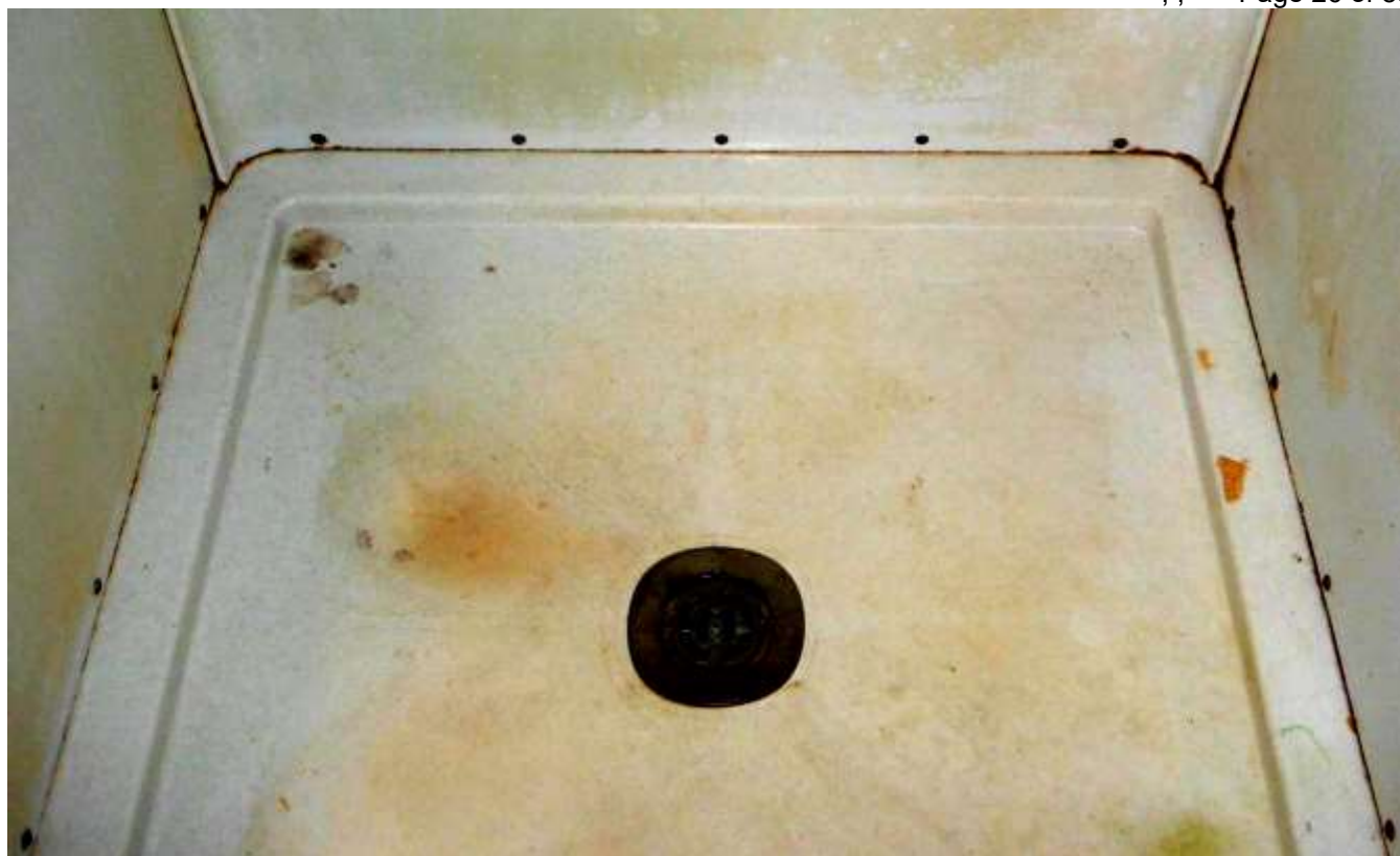
Figure 14 Recommend a bathroom contractor evaluate the bathroom and advise on all upgrades. Low quality/poor shower stall; rusted, stained, etc.
