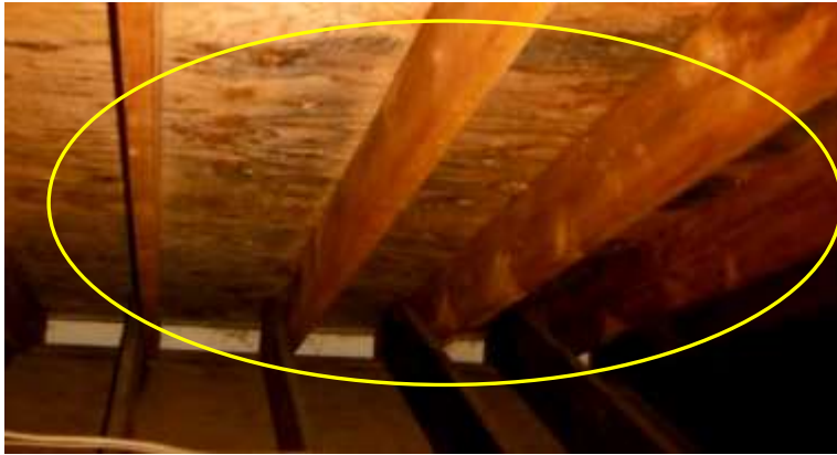
Figure 43 Example of mold like staining in attic; have affected plywood evaluated for replacement.
