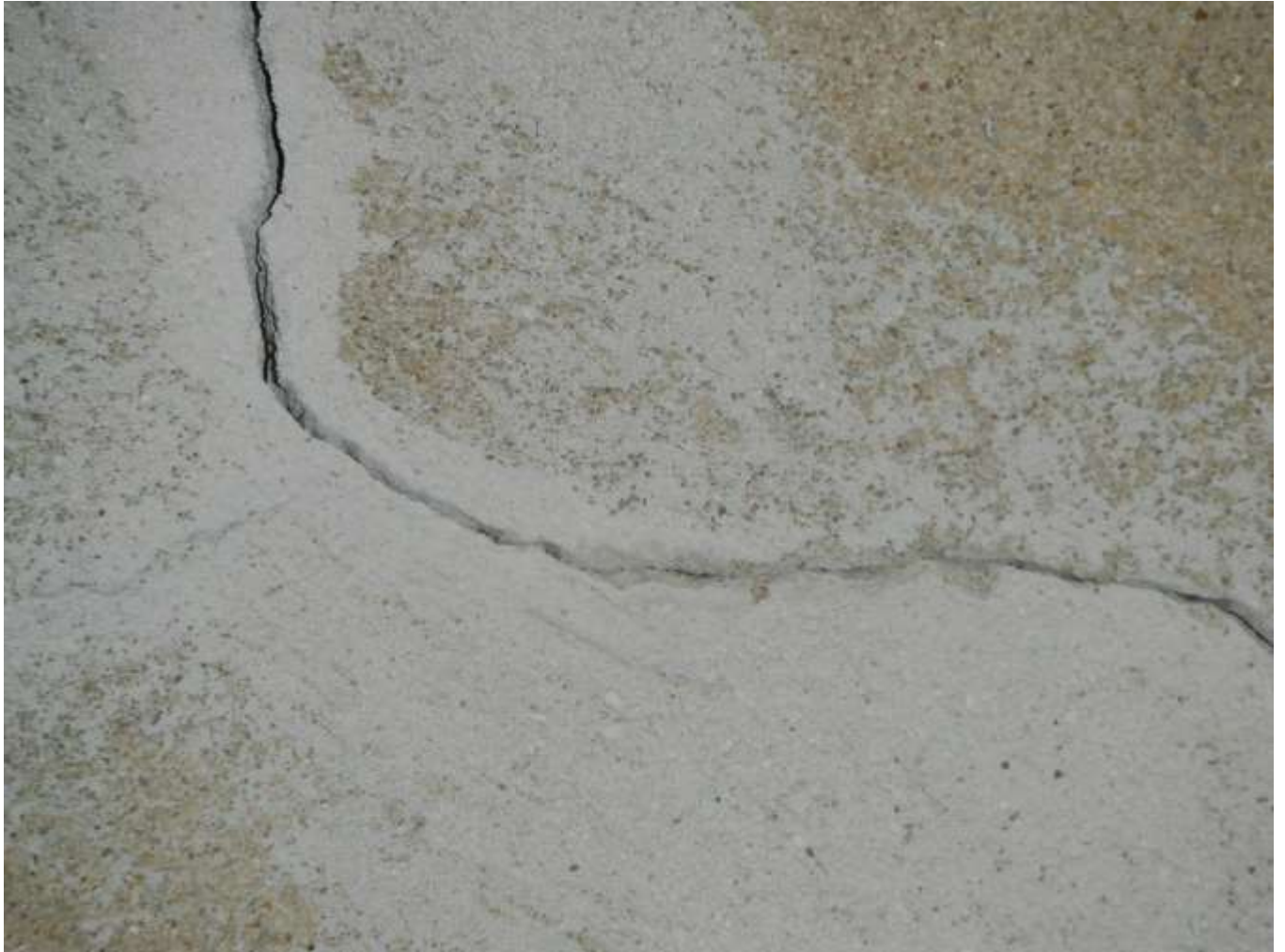
Figure 32 Foundation cracks; have foundation contractor, engineer or building contractor evaluate all foundation cracks and make repairs.
