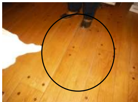
Figure 15 Have humps/warped boards/structure evaluated by contractor or engineer.
