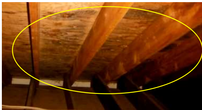
Figure 19 Example of mold like staining in attic; have affected plywood evaluated for replacement.
