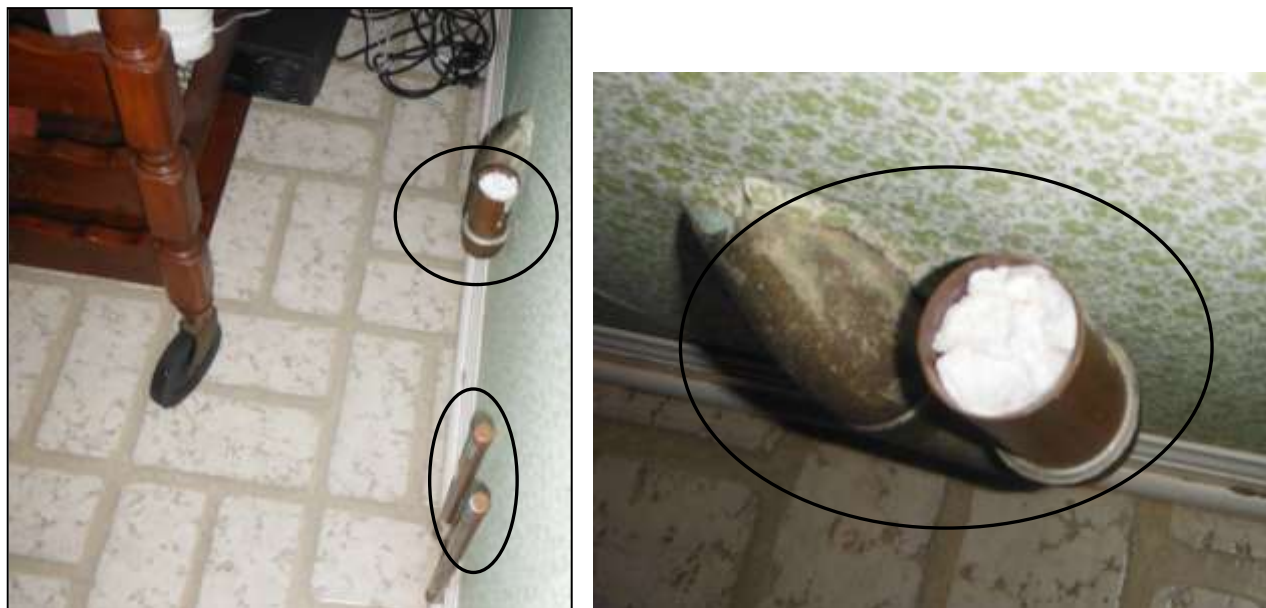
Figure 16 Drain with rag inside; have plumber cap off or remove all plumbing from below.
