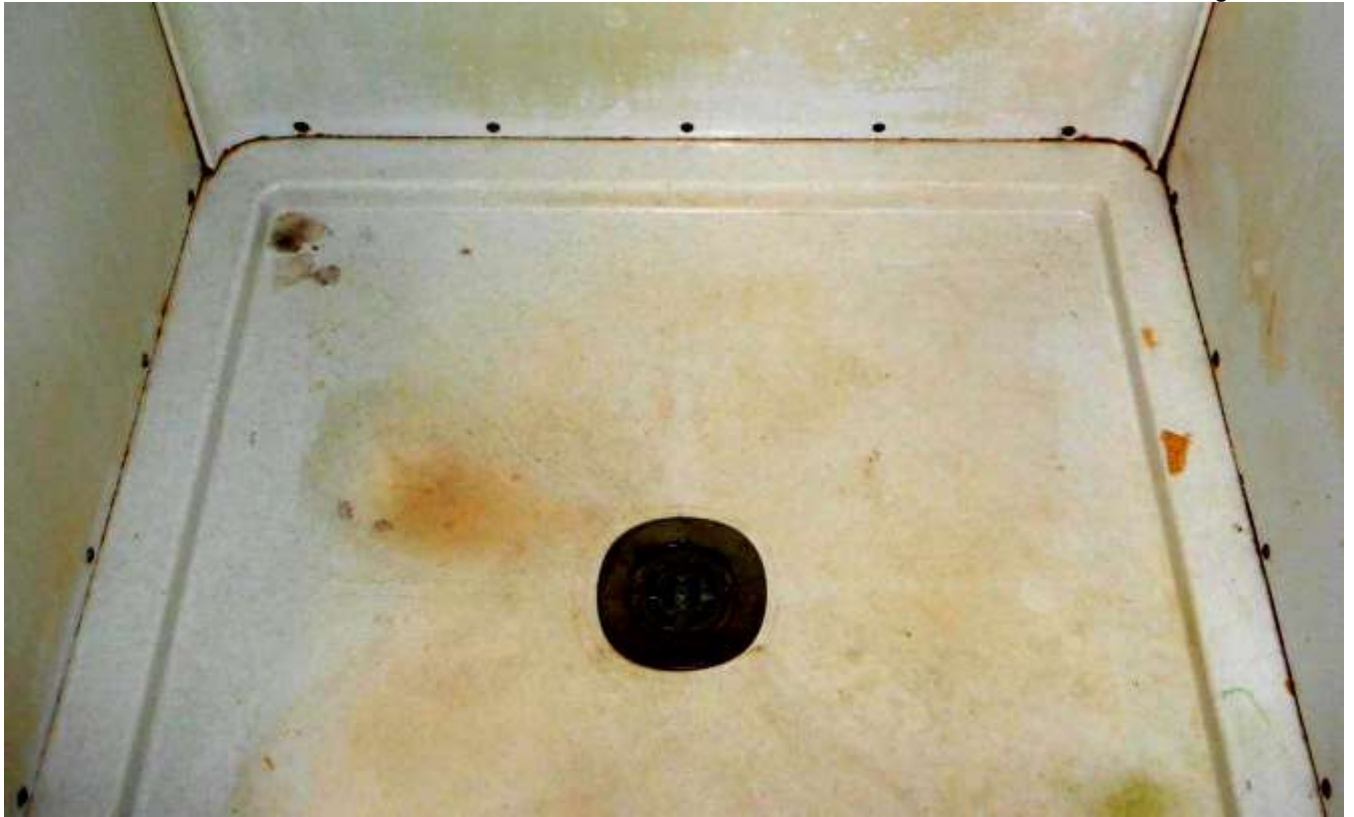
Figure 38 Recommend a bathroom contractor evaluate the bathroom and advise on all upgrades. Low quality/poor shower stall; rusted, stained, etc.
