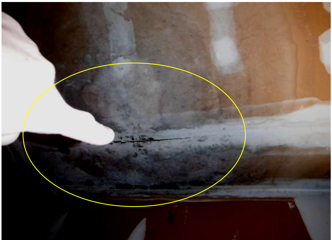
Figure 34 Example of roof leaking & water damage in garage. Have a structural carpenter evaluate extent of all damage including water, mold & insect before closing. The home was poorly maintained and needs upgrades and repairs everywhere.
