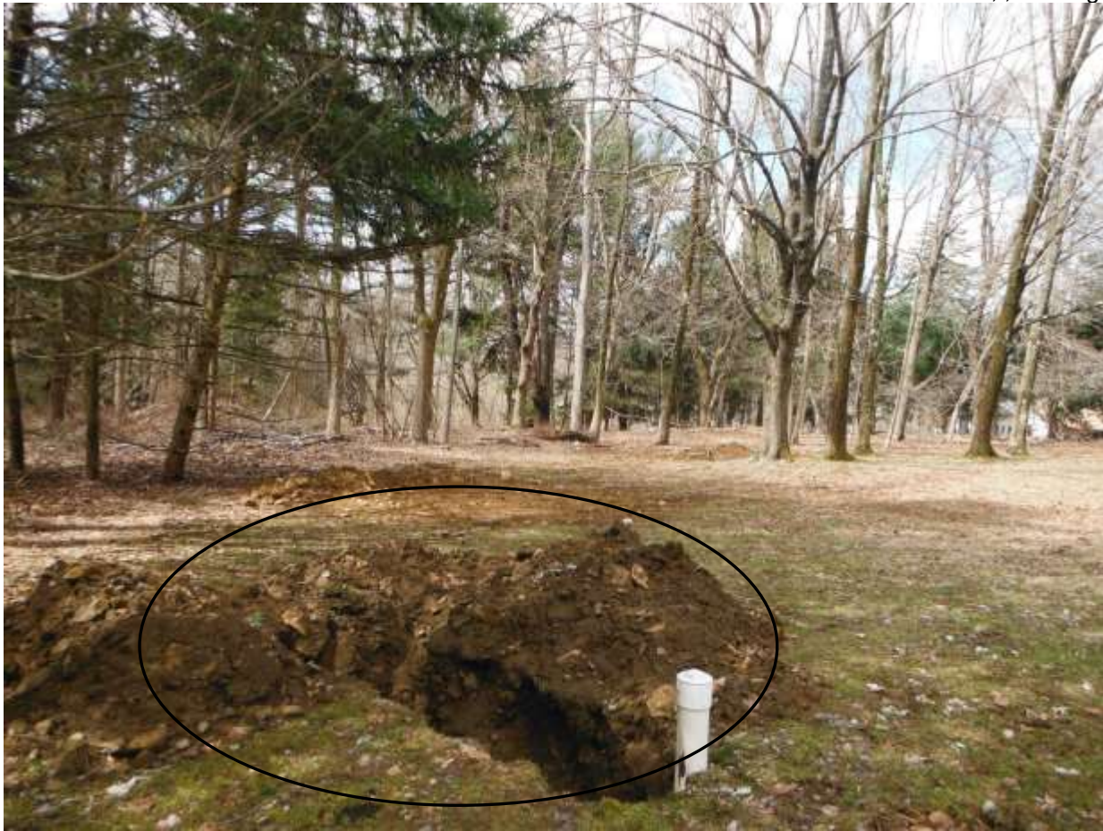
Figure 22 Open cavity for septic work or testing; fall hazard. Recommend fencing around open pit.
