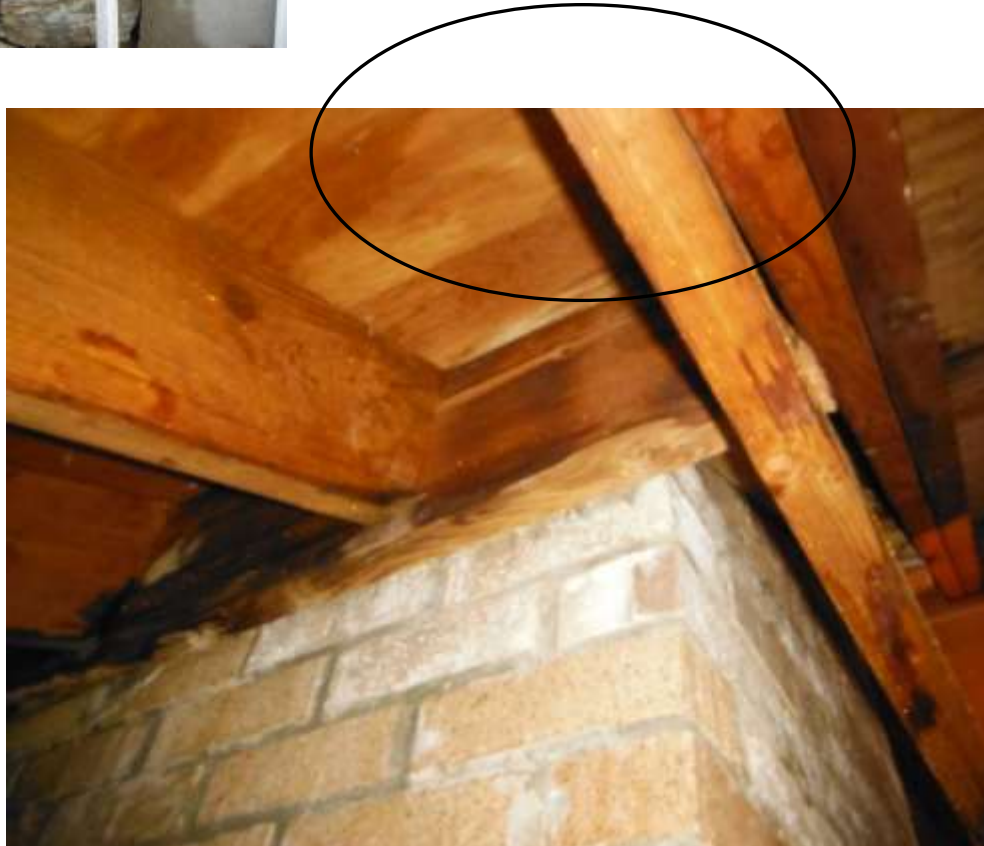
Figure 27 Leaking and efflorescence around chimney; view in attic.
