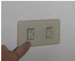
Figure 48 Have these switches evaluated; unknown what they control.
