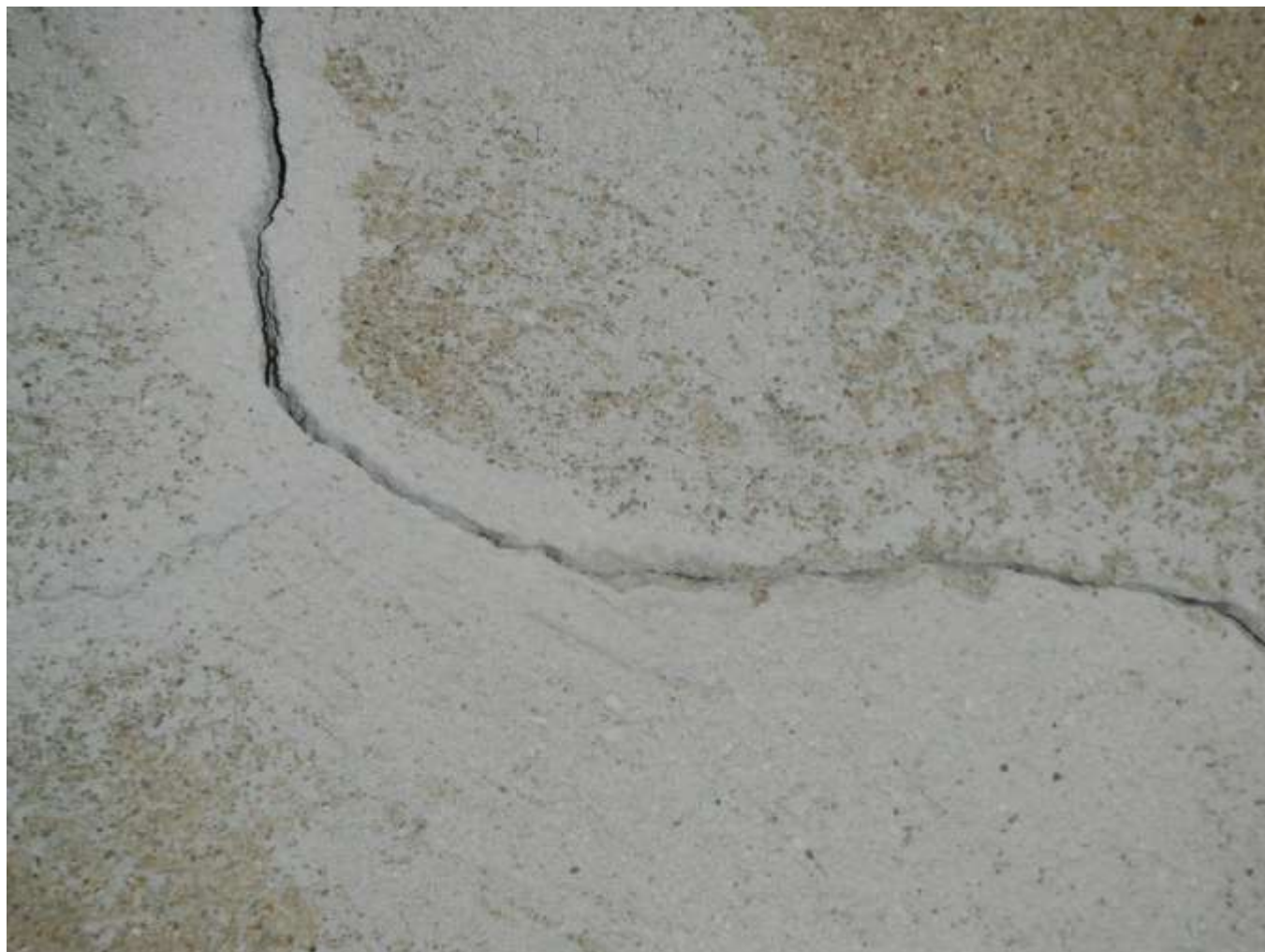
Figure 8 Foundation cracks; have foundation contractor, engineer or building contractor evaluate all foundation cracks and make repairs.
