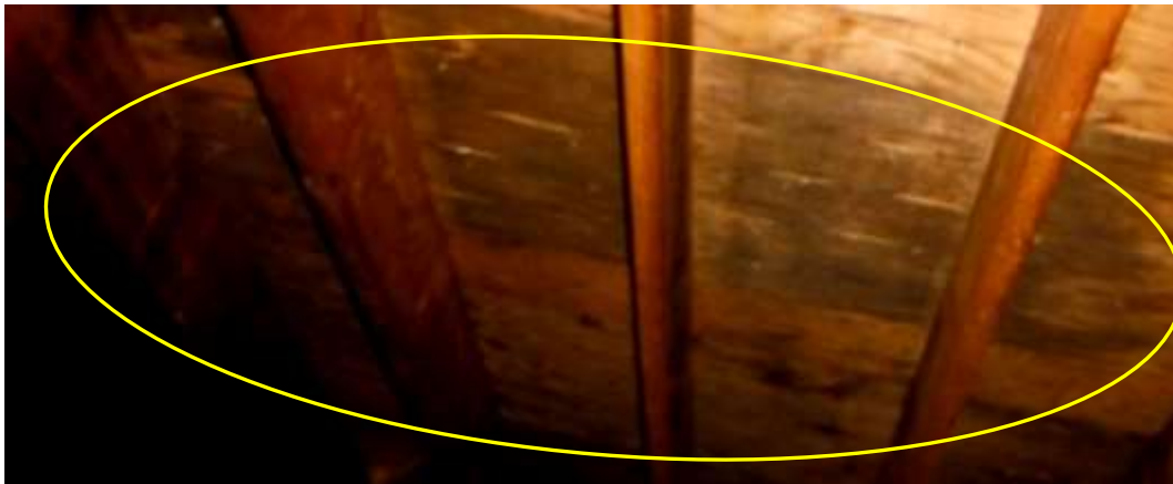
Figure 44 Example of mold like staining in attic; have affected plywood evaluated for replacement.
