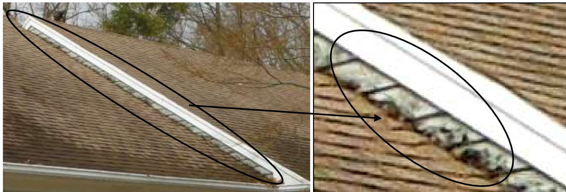
Figure 30 Rot on siding side wall/rook junctures.
