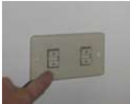
Figure 24 Have these switches evaluated; unknown what they control.
