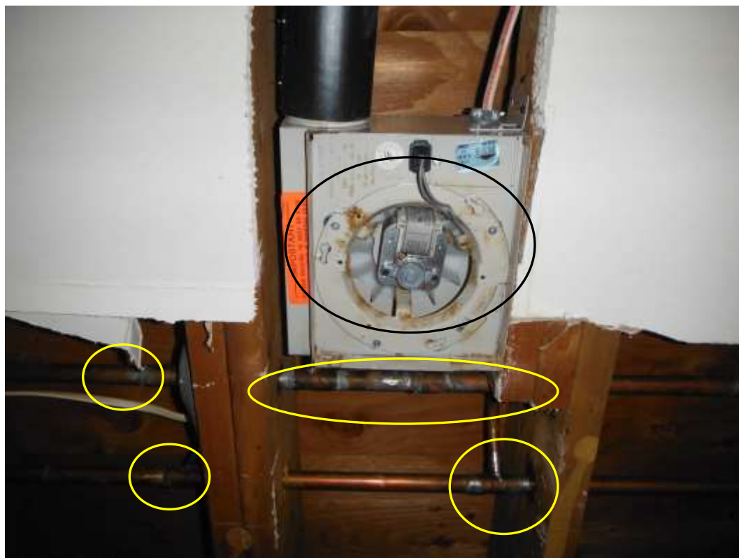
Figure 13 Opened ceiling and plumbing repairs; indication of frozen pipes/leak repairs. Have a bathroom contractor evaluate bathroom and upgrade with required permits.
