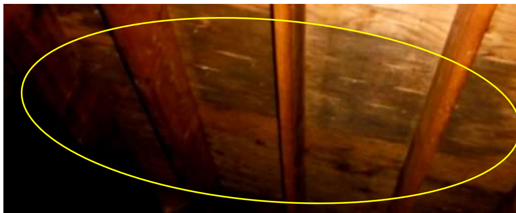
Figure 20 Example of mold like staining in attic; have affected plywood evaluated for replacement.
