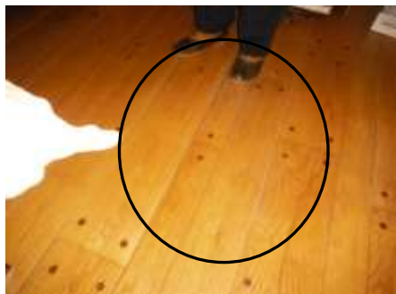
Figure 39 Have humps/warped boards/structure evaluated by contractor or engineer.
