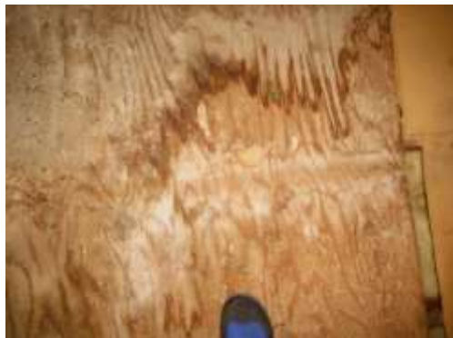
Figure 28 Water stains/leaking into attic.
