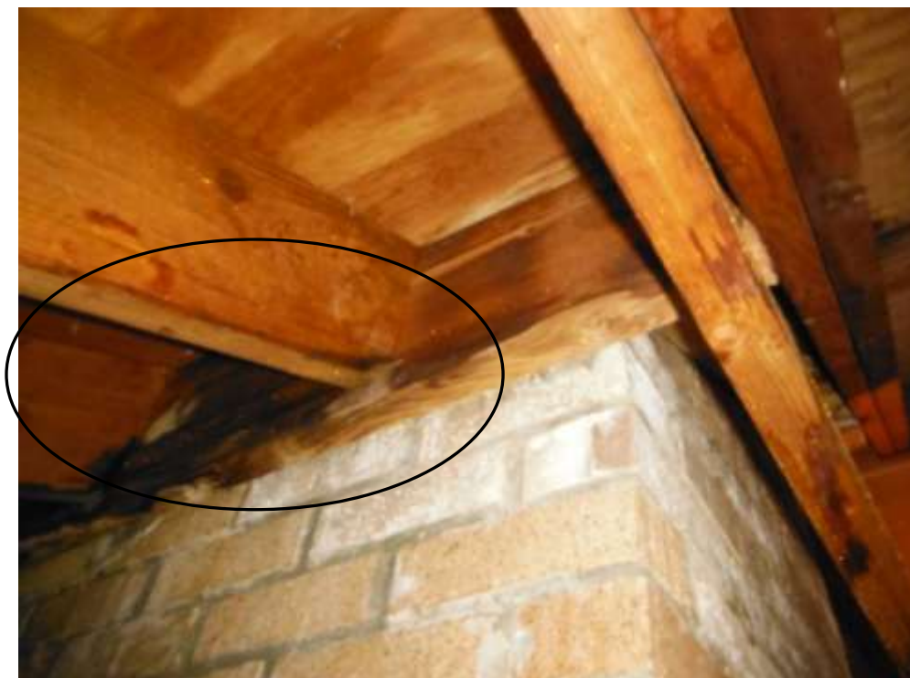
Figure 3 Leaking and efflorescence around chimney; view in attic.
