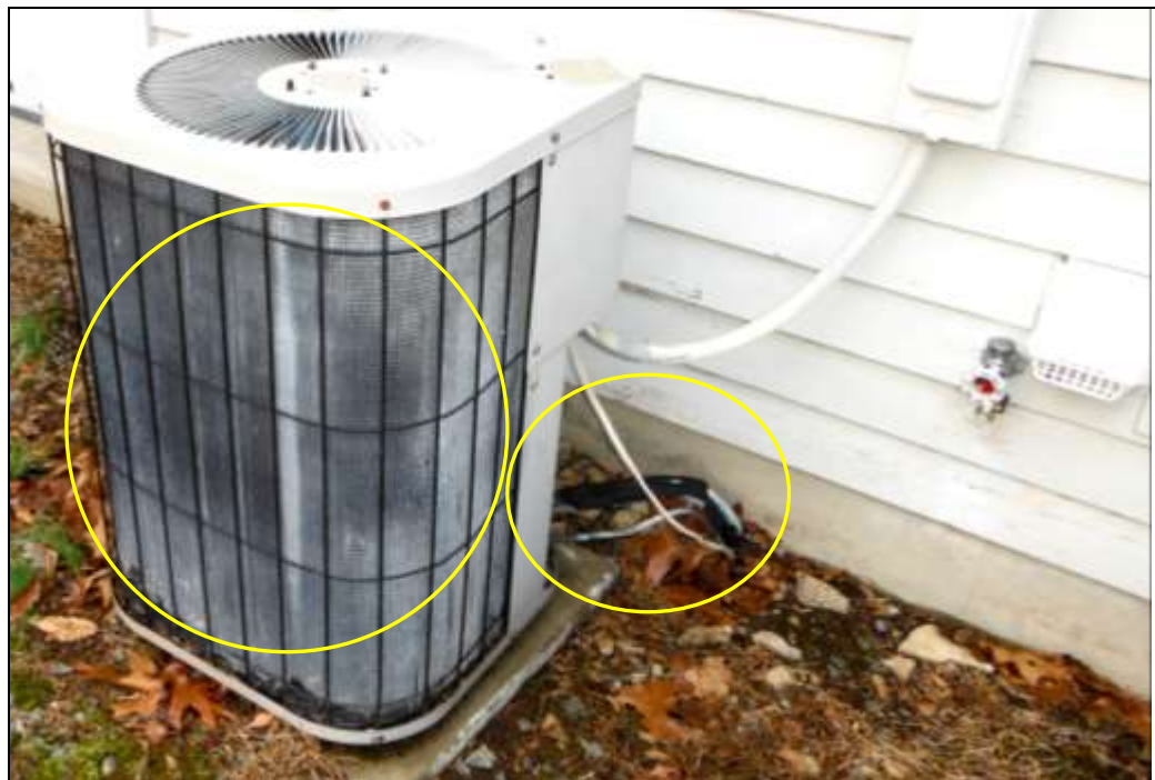
Figure 23 A/C past life & poor condition; damaged/flaking/oxidized fins, rust and corrosion, damaged insulation, etc.; have HVAC contractor evaluate the HVAC (heating & cooling) systems for replacements.
